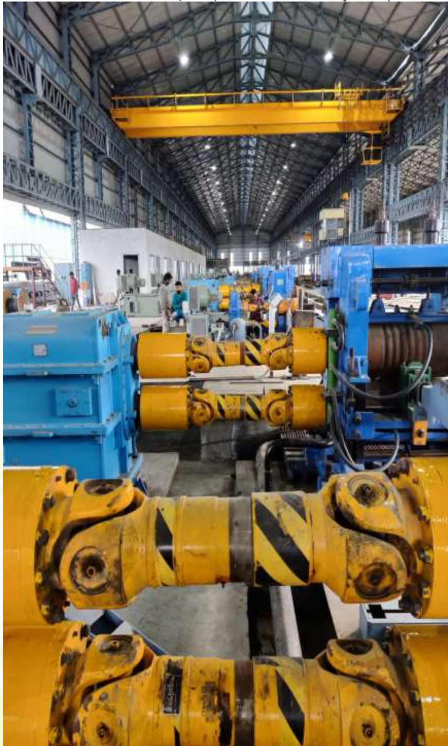
Figure 1.1: Actual photograph of Rolling Mill
