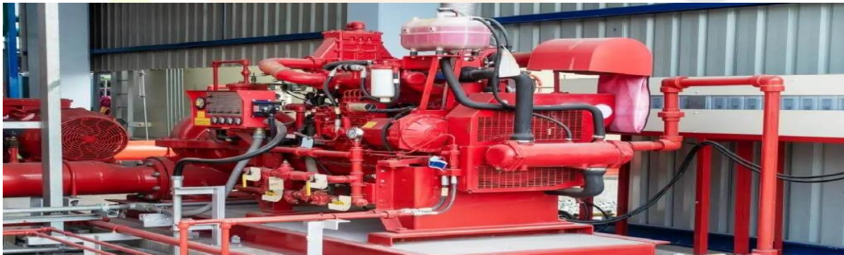
Fig. 4 Diesel Generator pump
