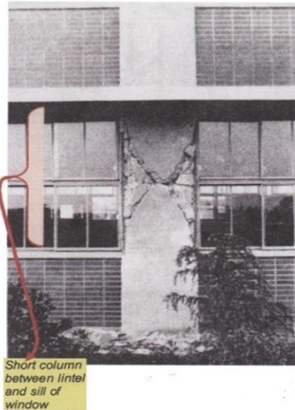
Figure-5 Short column between lintel and sill of window
