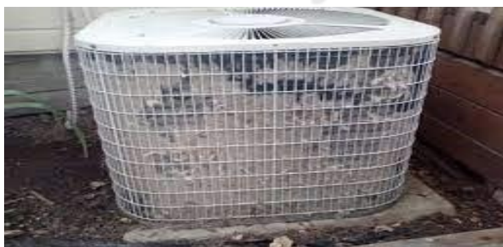
Figure 3: Dirty HVAC System
