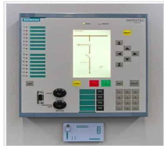
A digital (numeric) multifunction protective relay for distribution networks. A single such device can replace many single-function electromechanical relays, and provides self-testing and communication functions.
