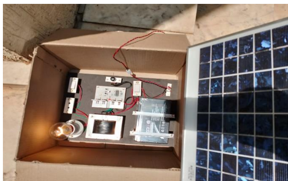
Fig ii) Circuit kit after Turn ON changing bulb glow and speed of induction motor in power system.
