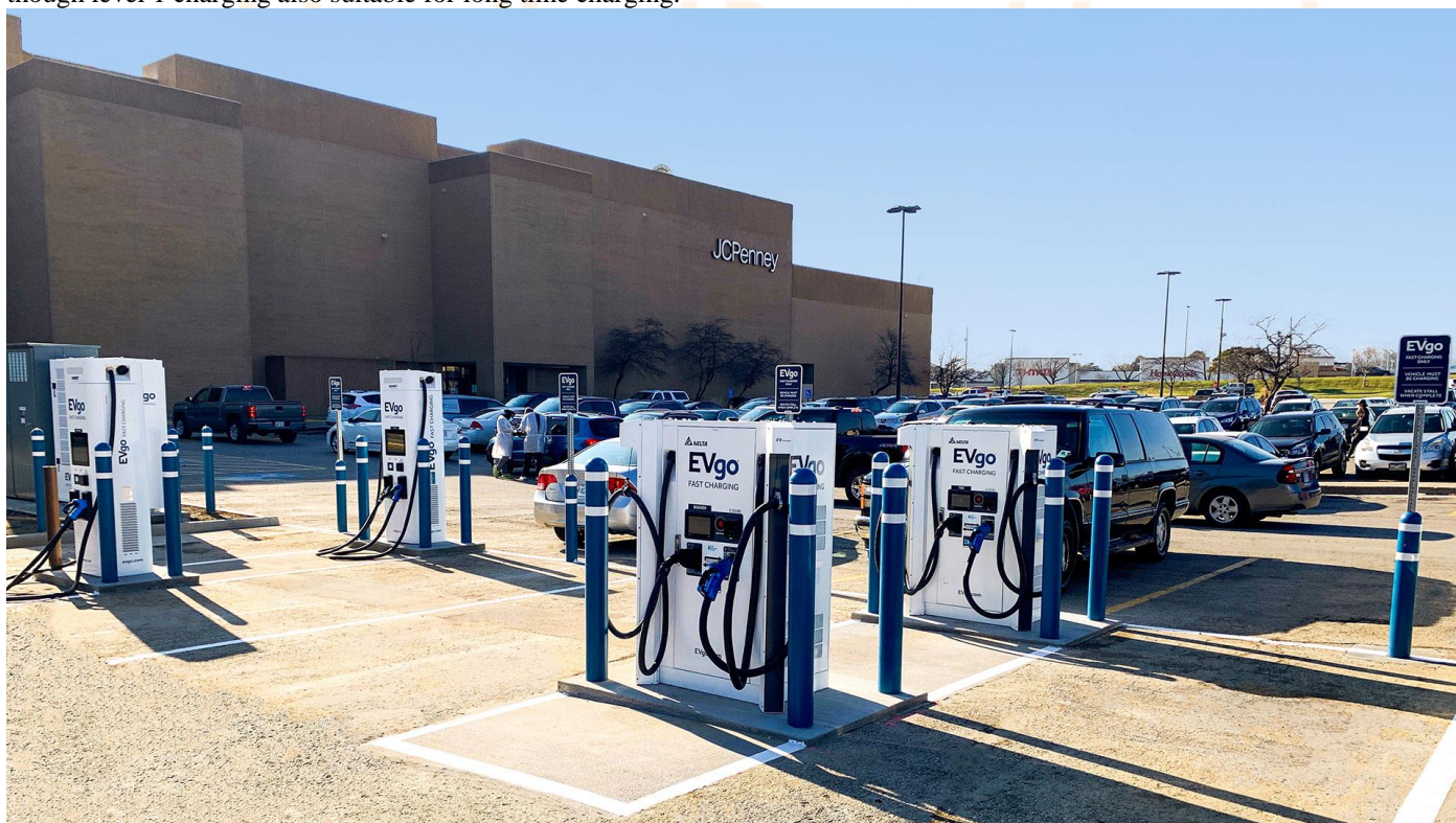
Fig. 7. EV charging station installed in Public places
